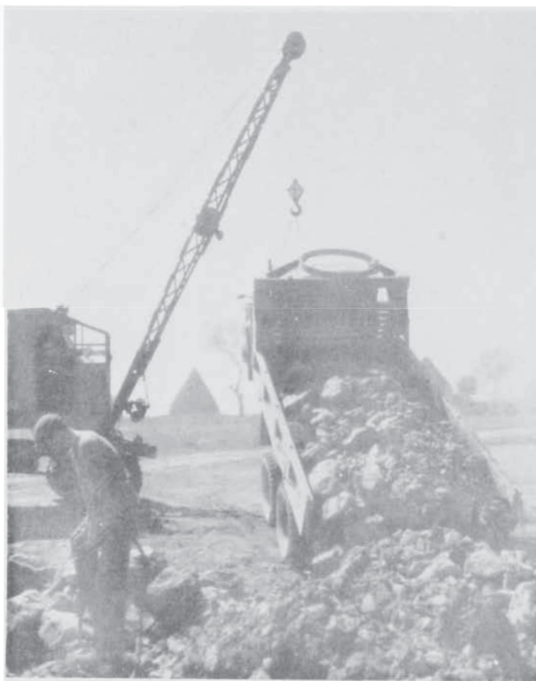
CRANE PLUS GMC EQUALS DUMP TRUCK FOR THE 16TH ENGINEERS WORKING ON NERO'S PIKE NEAR ANZIO
